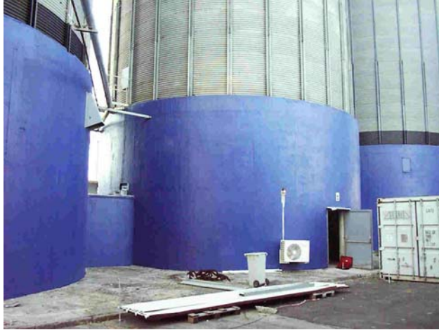
Metallic silo with concrete foundations and metal anchorage rods in the soil being used as a natural earthing system
